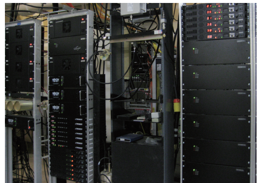
Communications room in large hotel where NEXEDGE® has been installed
